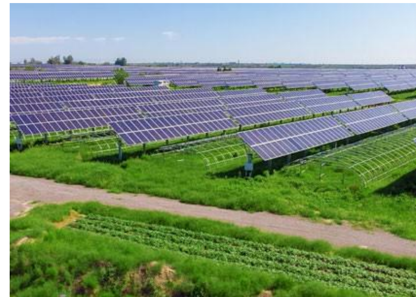
Fenglei Photovoltaic Power Station of Sinopec Star
