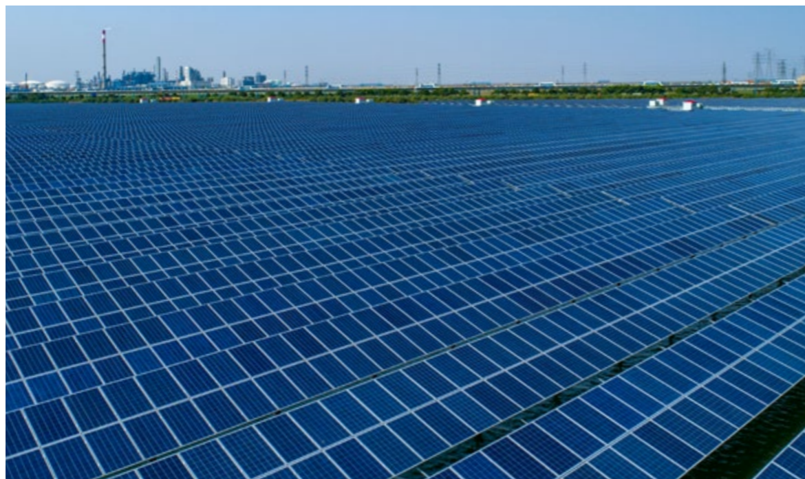
Pilot photovoltaic power generation project on a reservoir in Zhenhai Refinery
